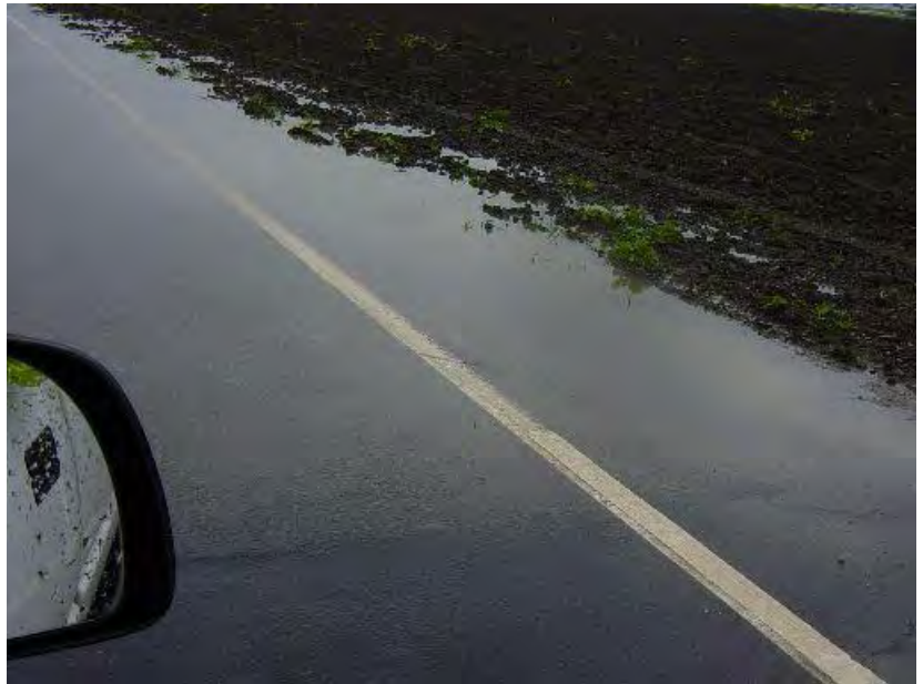
P18—Flooded area on Flynn Rd
