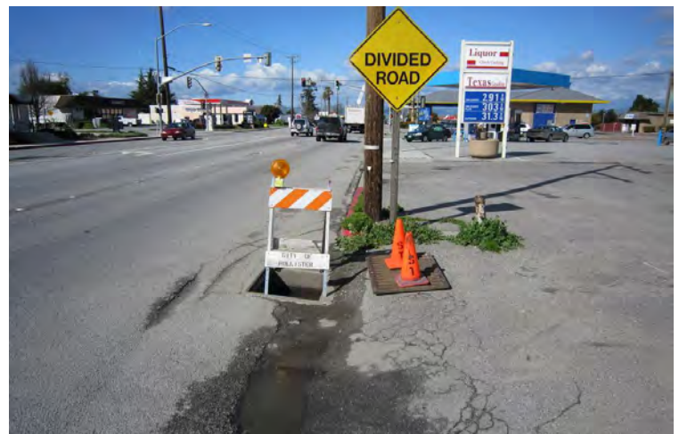
P16—Flooded area on San Benito from RR ditch
